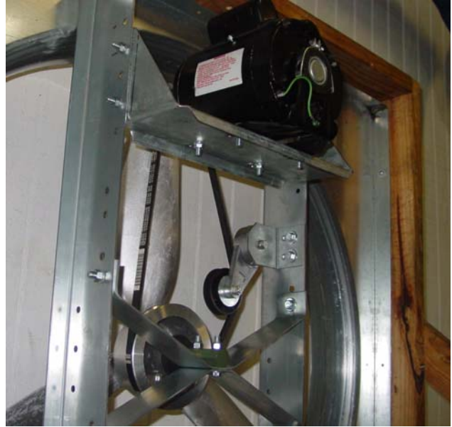
NBC36 with motor mounted at the top of the fan
